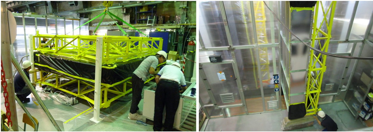
Figure 3.10: (left) Picture of the C0 section on the LSM mezzanine with its two support structures, before lowering to the SuperNEMO integration clean tent. (right) Insertion of the C1 section in the clean tent with C0 already inside.
