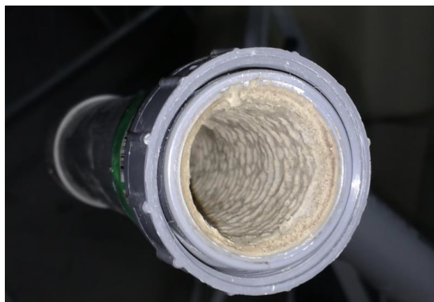
Figure 3.20: Mineral deposit inside a PVC pipe for urine diverting toilets. Source: Brun (2019)
