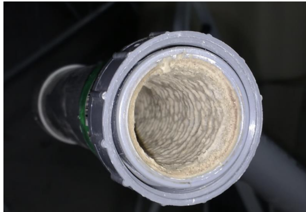
Figure 3.20: Mineral deposit inside a PVC pipe for urine diverting toilets. Source: Brun (2019)
