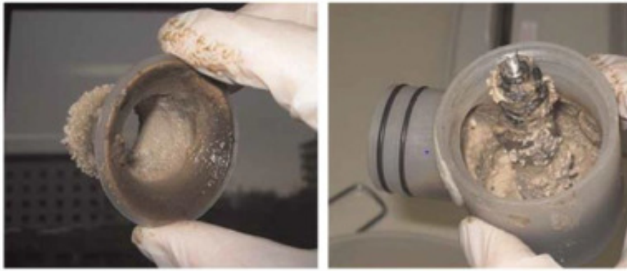
Fig. I.2 – Illustration of salt precipitations and subsequent deposits occurring inside collection systems (the pictures show a valve used in the “NoMix toilet” equipment from Roediger Vacuum GmbH) (extracted from [51]).
