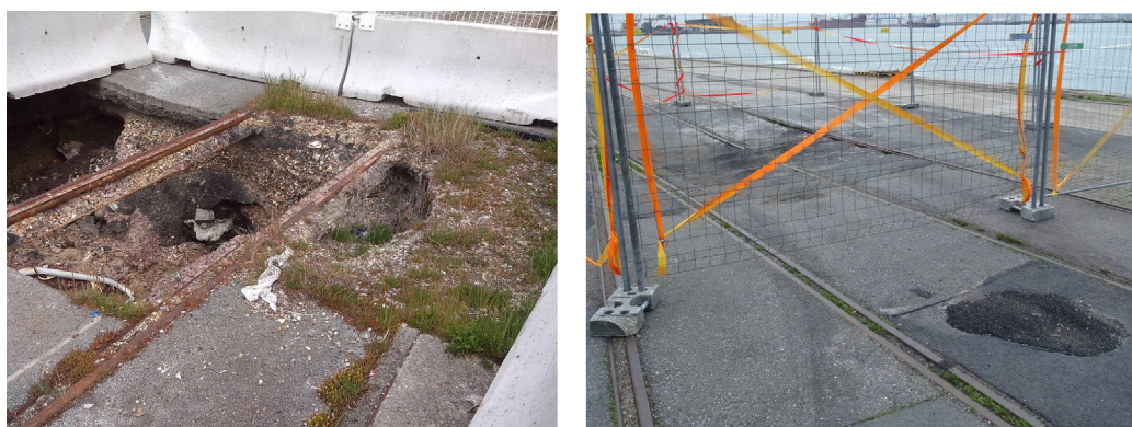
Fig. 2. Photo of typical collapse and deformation observed these last years on the Joannes Couvert quay.
