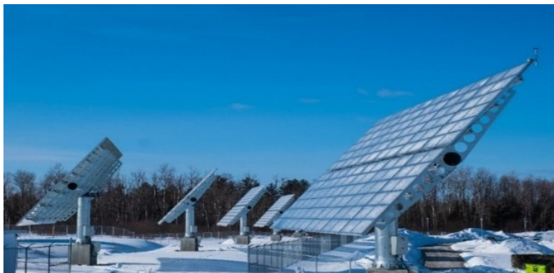
Figure 4.2 Five out of eight CPV systems in Université de Sherbrooke solar park, Quebec
