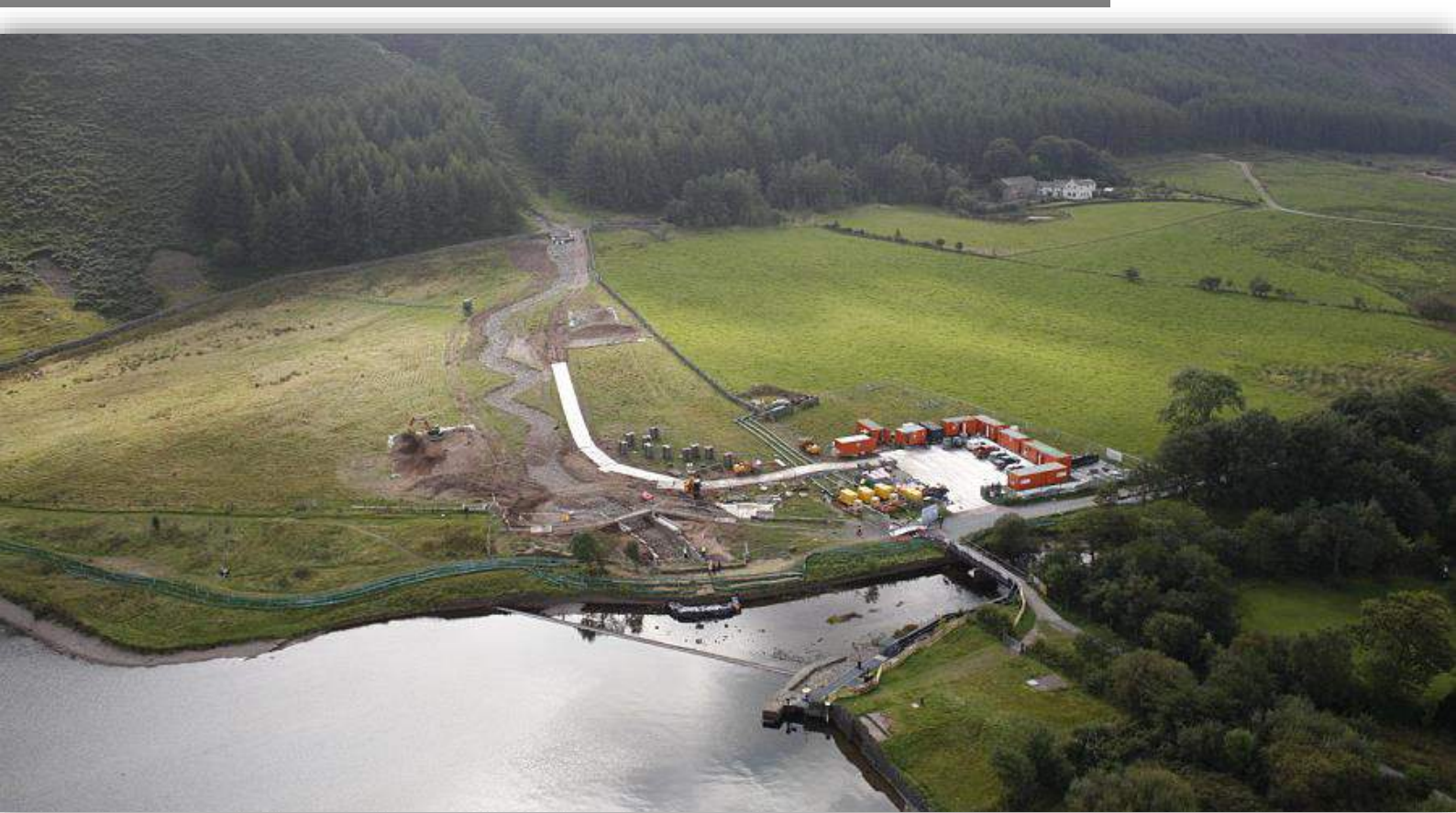
Outlet of Ennerdale Water during the engineering work undertaken to reconnect Ben Gill to the River Ehen. Photo: SUAVE Air Photos, September 2014.
