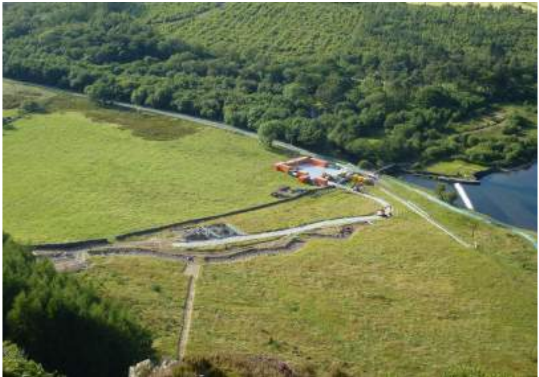
Plate 1.2. View from the fell of Ben Gill alluvial fan during the construction work of the new channel, summer 2014 (Photo: Baptiste Marteau).
