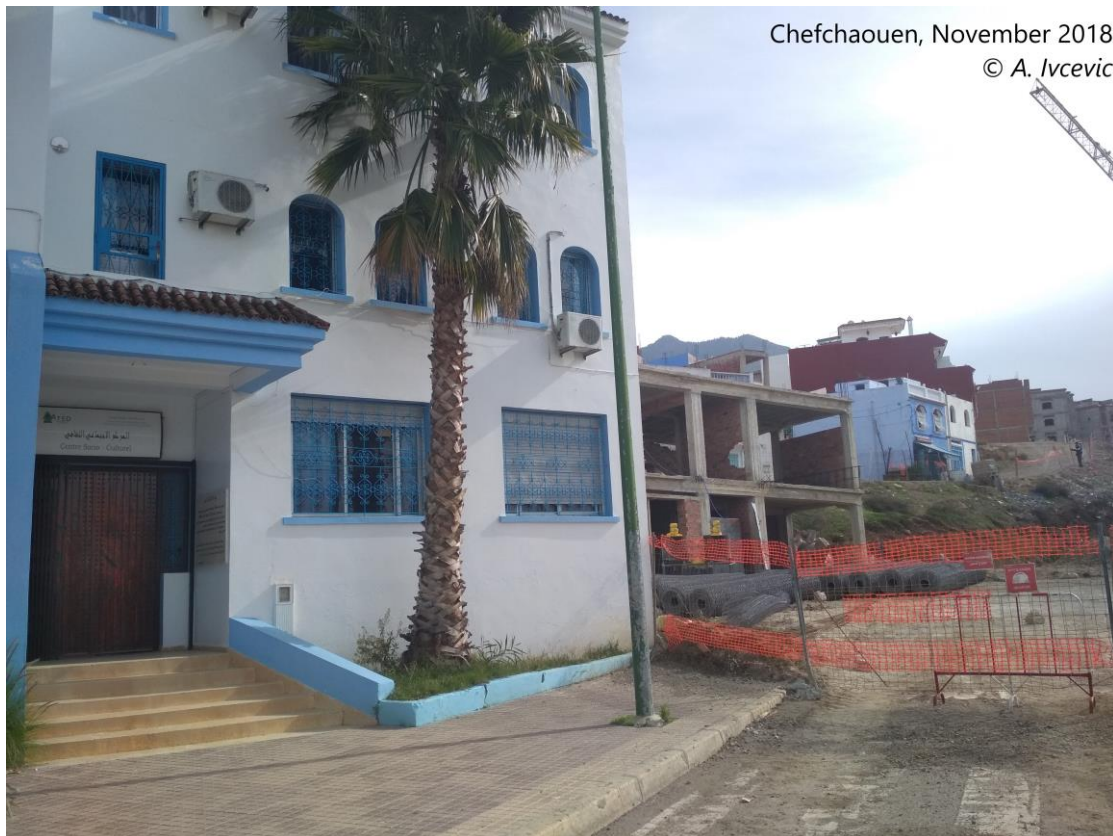
Figure 23: Landslide stabilisation works just in the neighbourhood of my interlocutor's association from Chefchaouen.
