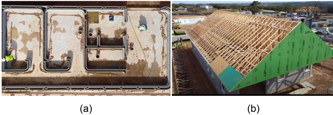
Figure 2.33 – The ICON-3D Printed House: Illustrating the Conventional Use of 3D Printing in Residential Construction with Roofs Constructed by Labour Force
