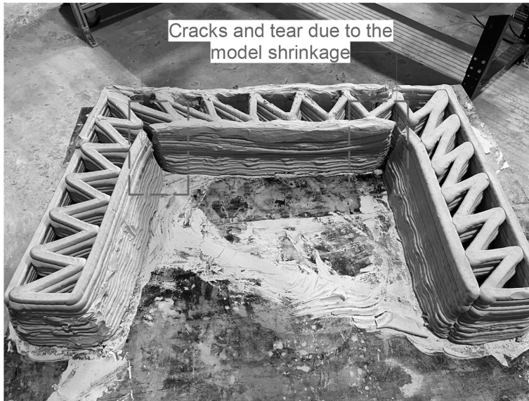
(b) U-Shape wall after shrinkage (dry)
