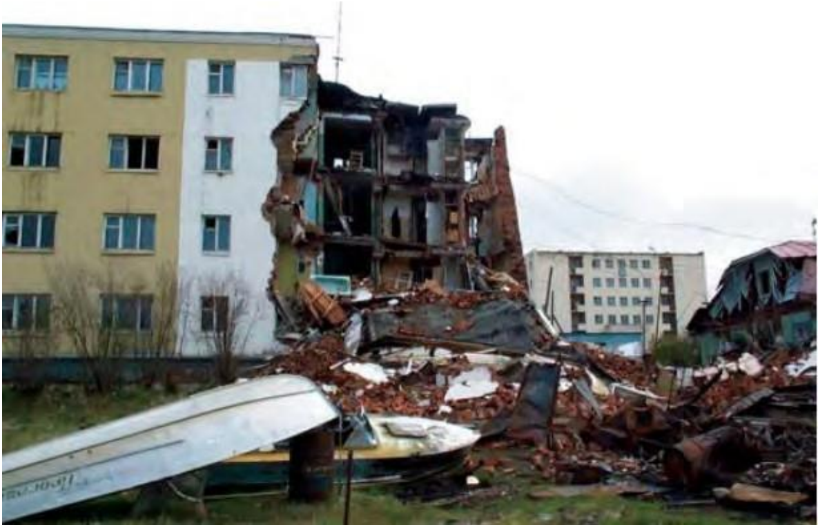
Figure 33: Part of a building in the town of Chersky collapsed in June 2001 due to the weakening of the foundation built upon permafrost.
