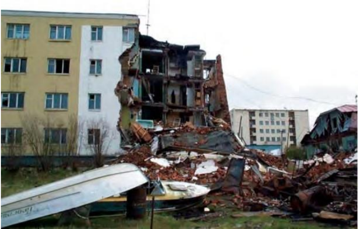
Figure 33: Part of a building in the town of Chersky collapsed in June 2001 due to the weakening of the foundation built upon permafrost.
