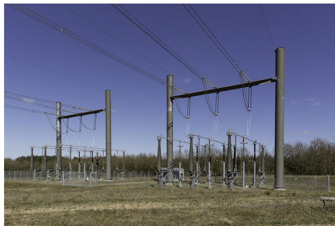
Figure 3.3: Transition station of the Kassø-Tjele 400 kV HVAC transmission line in Denmark [74].
