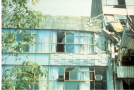
Figure 1.2: "Pounding damage at Hotel De Carlo" (Arnold, 1985)
