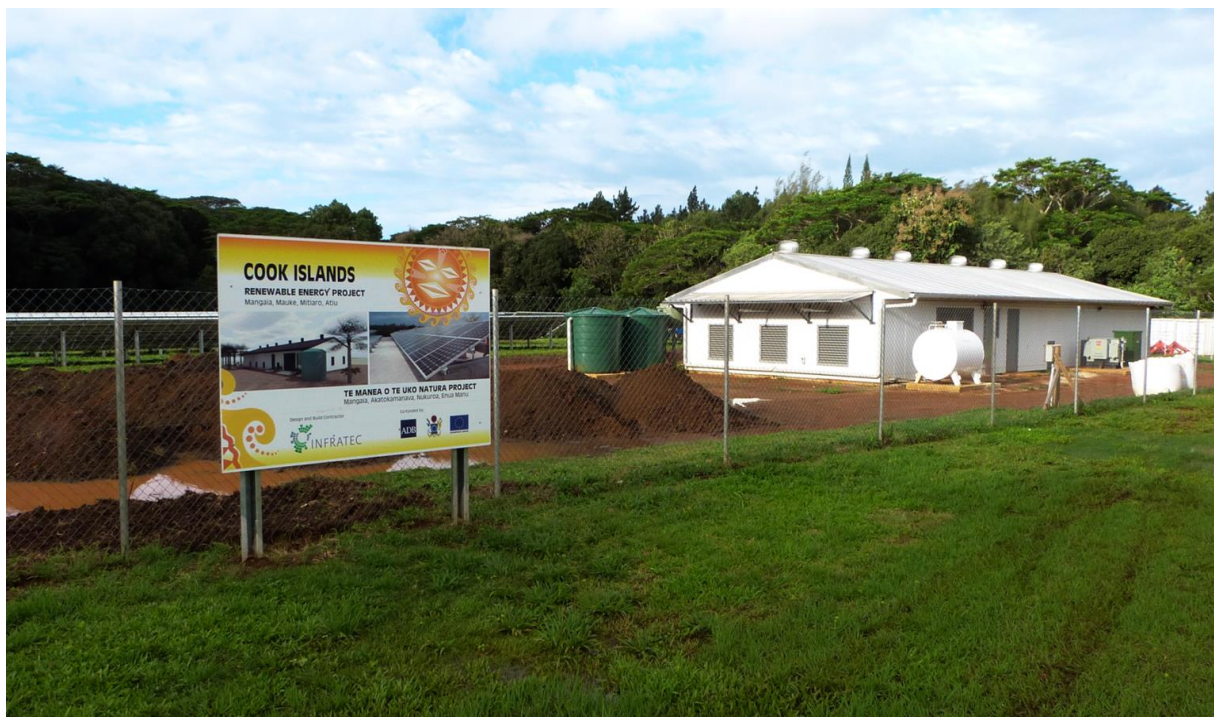
Figure 11 - Station solaire de Ma'uke (photo D. Glory, 2018)
