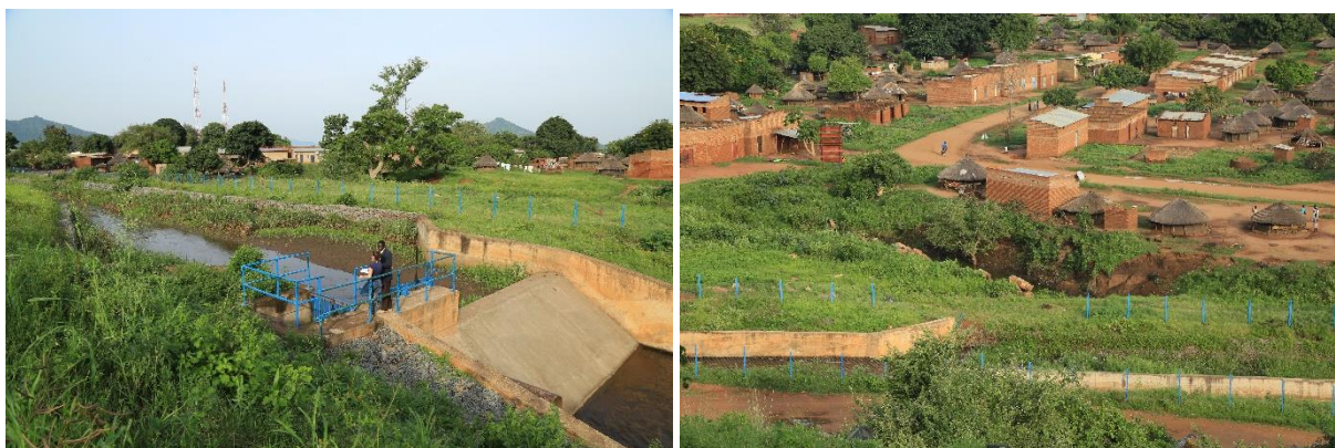
Picture 31 (left): Fenced, cemented dam diverting water to the spillway and underground pipeline at the end of the rainy season (Torretti 2016)
