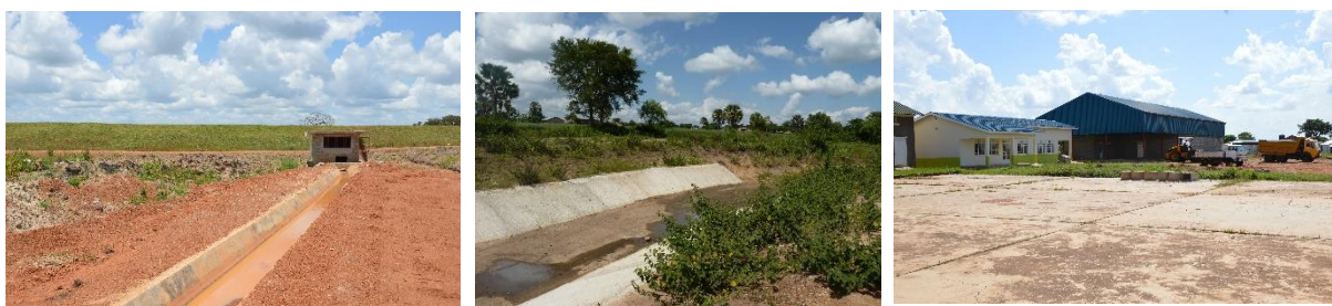
Picture 16 (left): Upgraded Itek main buffer dam and cemented water channel (Torretti 2016)
