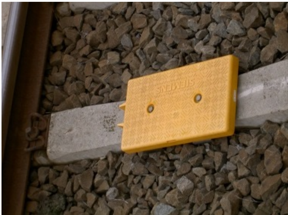
Fig. 2.22 Balise between the rails. (source: Wikipedia)
