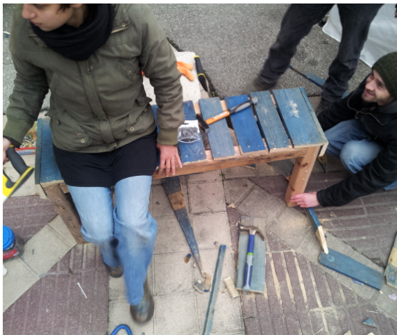
Figure 2.10 Constructing the bench that served as a transitional object between Villeneuve and the Institute of Urbanism and Alpine Geography. (Photo Planning, May 2014)
