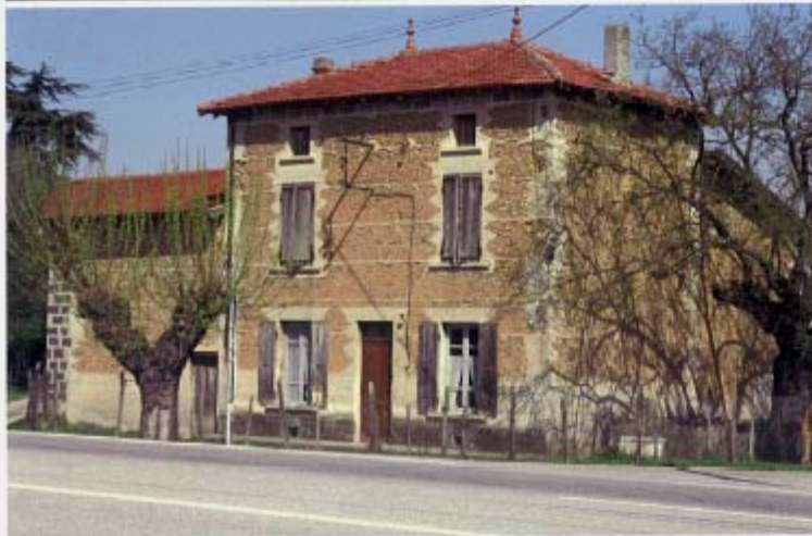
b: A typical village house in "pisé", built at the beginning of the XX e Century, with reveals in concrete, located in the northern part of Dauphiné, region of Isere, South-East of France. Most of these houses are not plastered though the local climate is very rainy in Spring and Autumn. The main front façades of wealthier houses are sometimes decorated with layers of burnt bricks and river pebbles.
