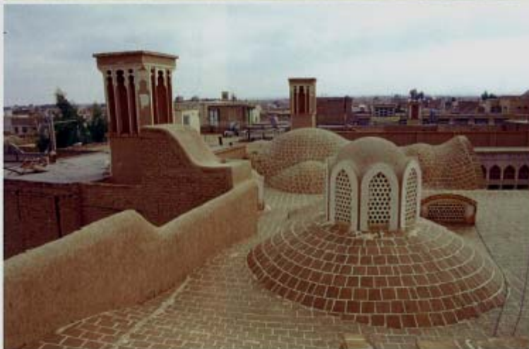
b: The climatic adaptation of the earthen architecture in Iran has produced the famous tradition of the wind towers or "badgales" which can be still observed in the desertic region of Yazd (Central Iran) and in numerous other regions suffering of a very hot climate in summer. Here, such bioclimatic devices are observed on the roofs of the "Frigeritha house", located in Kashan, one of the jewels of the Kajar architecture (end of the XIX e Century and beginning of the XX e Century).
