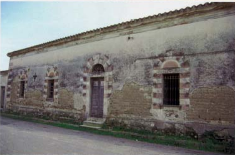
b: Typical house in unbaked earthen bricks, "ladriri" or "mattoni", in southern Sardinia, region of the "Campidanu", village of Riola Sardo. In this region, numerous villages are built in earth and a programme for their conservation, restoration, rehabilitation and maintenance, associated to a revival of the earthen building technology has been recently launched under the guidance of the University of Cagliari in close collaboration with the municipalities. This tradition of the unbaked earthen brick traces back to Greek, then Punic (site of Tharros) and Roman times.
