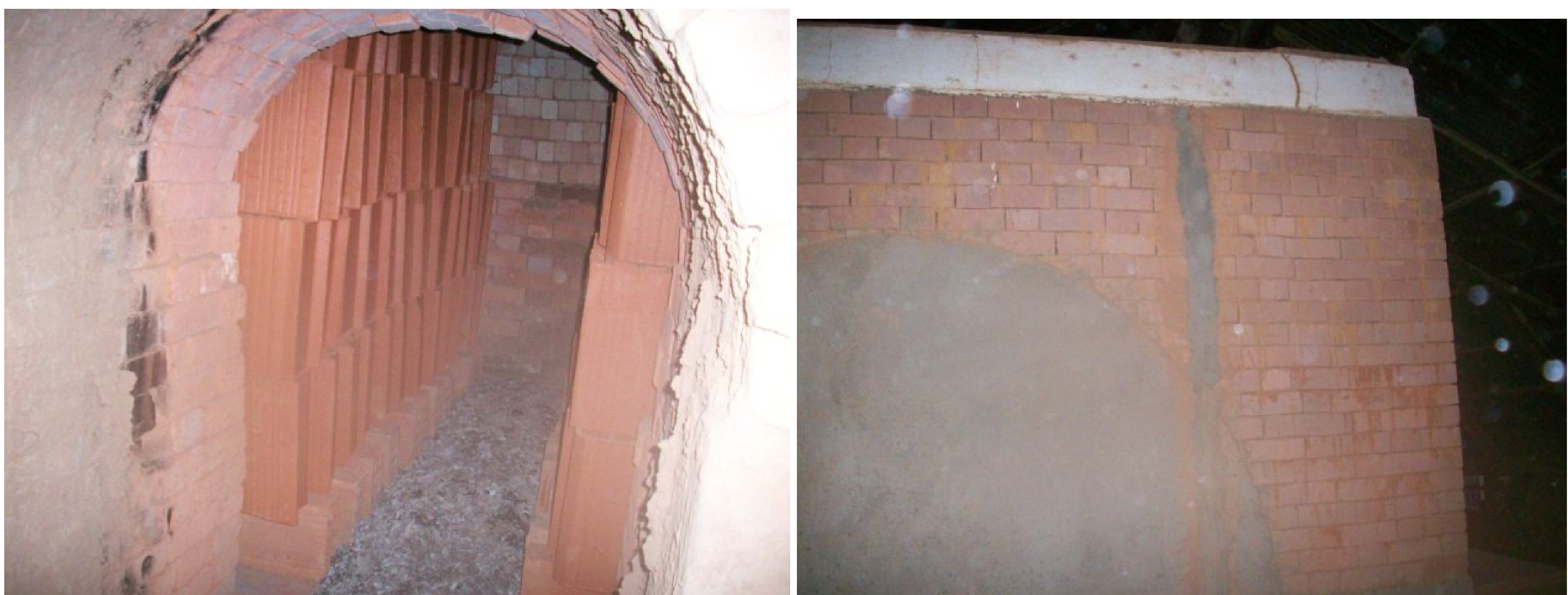
Figure 16: Four semi-industriel (briqueterie d'Ambohimena).
