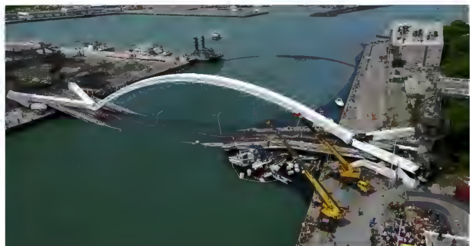
Arch Bridge collapse in Taiwan Bay (1/10/2019).
