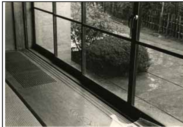
Sliding doors in Japanese room with floor heating grid on the left (1F)
