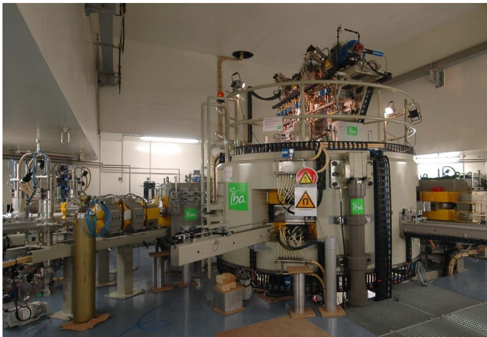
Figure 3.1 Le cyclotron ARRONAX en casemate centrale (CC).
