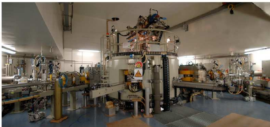
Figure 3.3: IBA ARRONAX Cyclotron in the principal bunker.
