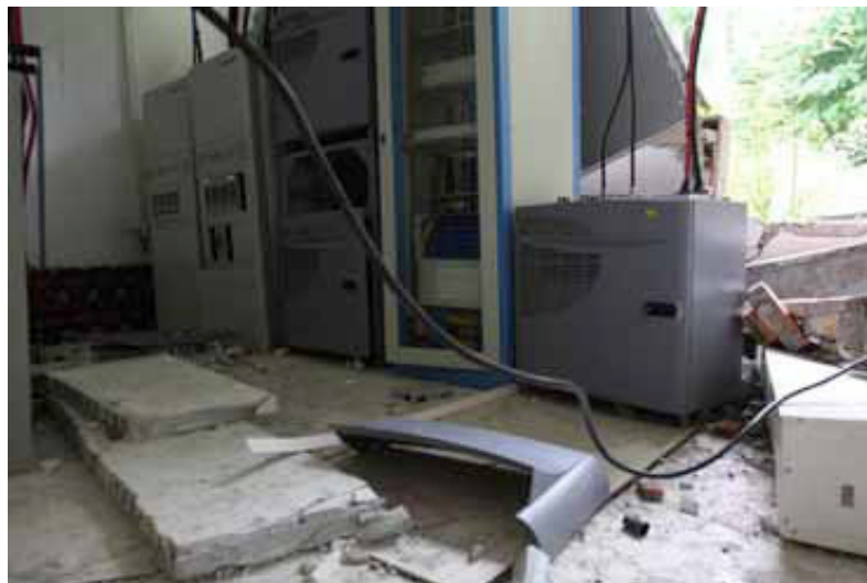
Figure 50. Ming et al. (2008). “Outside wall of the communication machine room, inward collapse”.
