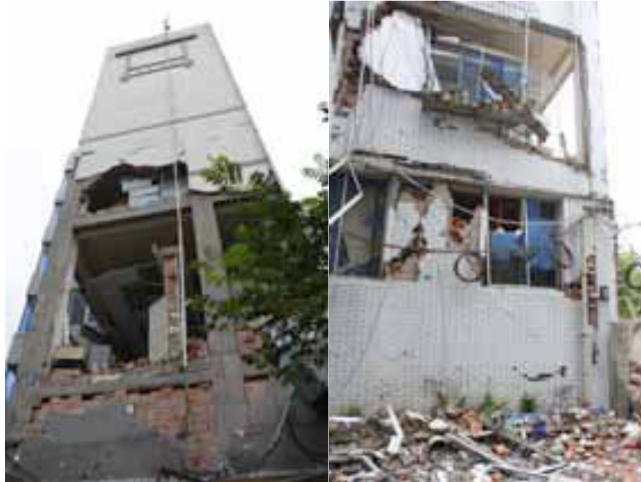
Figures 51 and 52. Ming et al. (2008). “Outside cross walls and cables damage of three floors of the traffic administrative bureau.”
