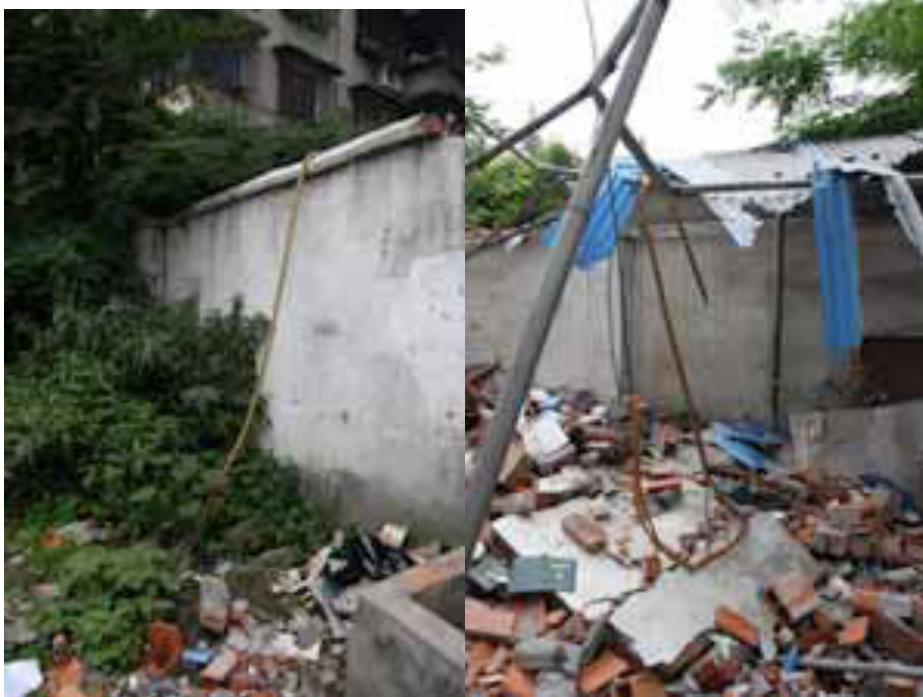
Figures 48 and 49. Ming et al. (2008). “Broken optical fiber cable that ran across enclosing walls.” 443
