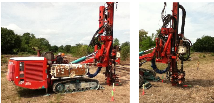
Figure 4-4 Casagrande C4 drilling rig used to install the soil-cement columns in Vernouillet
