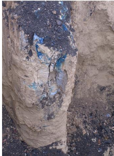
Figure 4-52 Cracks and fissures observed on column C2 approximately 1 m below ground level.
