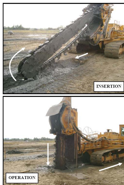
Figure 1-9 Insertion of the mixing blade and operation of the Trenchmix method (Lebon, 2005).
