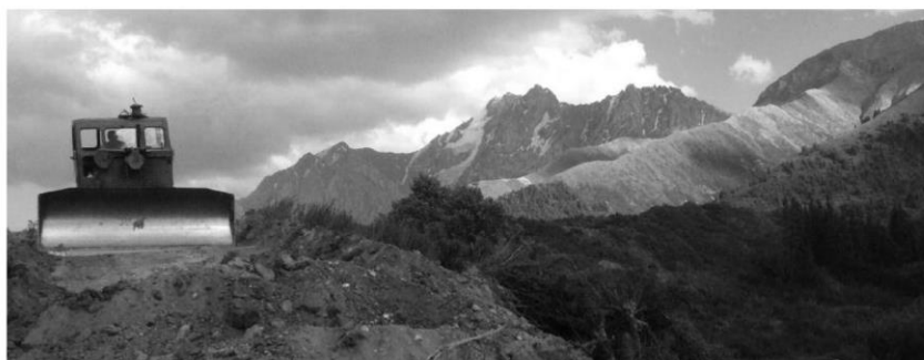
Figure 4. Renovation work conducted by the PC of Žerge-Tal on the road leading to the remote pasture of ǝng Ta (built during the Soviet period), 20/08/2013
