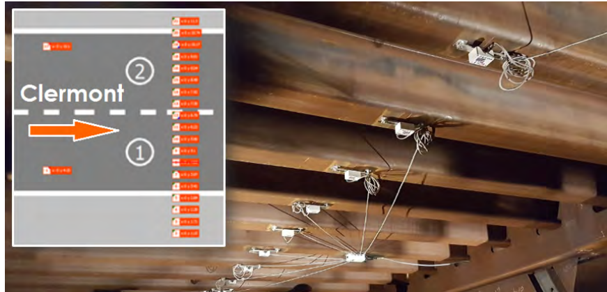
FIGURE 3.6 – BWIM system, scheme and photo inside the deck of the viaduct
