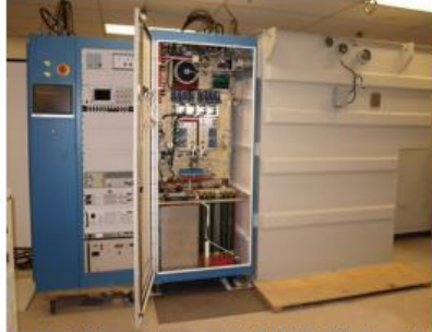
Figure 1. DTI's prototype solid-state ESS-class klystron modulator, developed under a DOE SBIR grant. This design is optimized for long pulse operation with highest possible reliability and availability required for particle accelerator user facilities and test stands.
