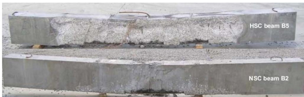
Figure 2.14: Fire spalling of normal strength concrete (NSC) Beam B2 (SF and load of 50 kN) and high strength concrete (HSC) Beam B5 (LF and load of 60 kN) [44].
