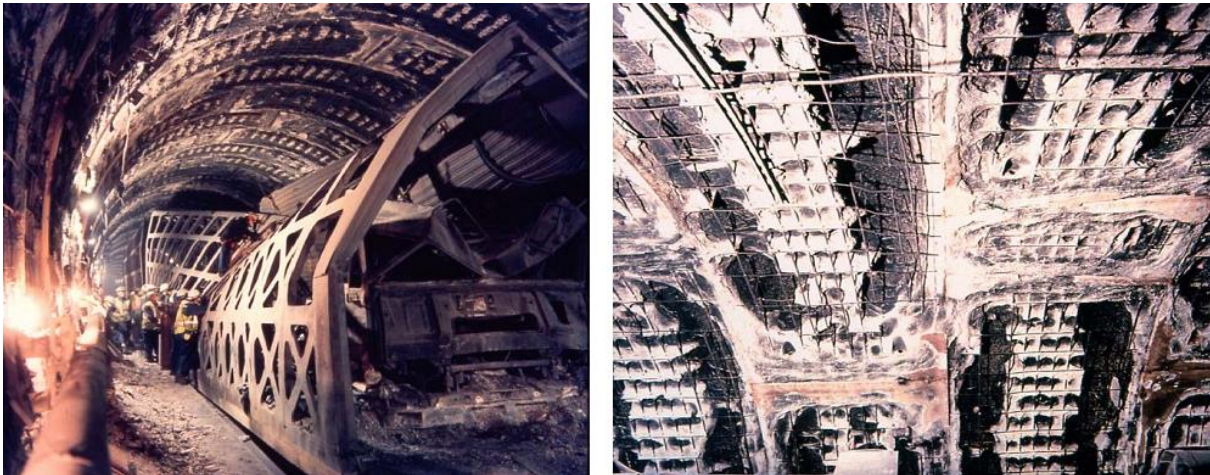
Figure 1.1: Damage in the lining of the Channel Tunnel between France and England after the fire accident on November, 18 th 1996.
