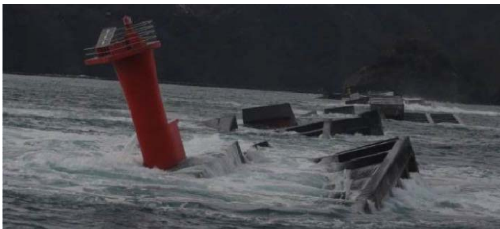
Figure 1.8: Damages in the north part of the Kamaishi breakwater.
