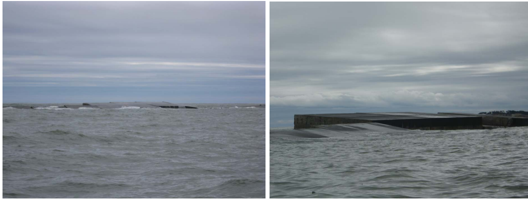
Figure 1.7: Caisson displaced in the offshore breakwater of the Port of Soma (from Tsimopoulou (2011) ).
