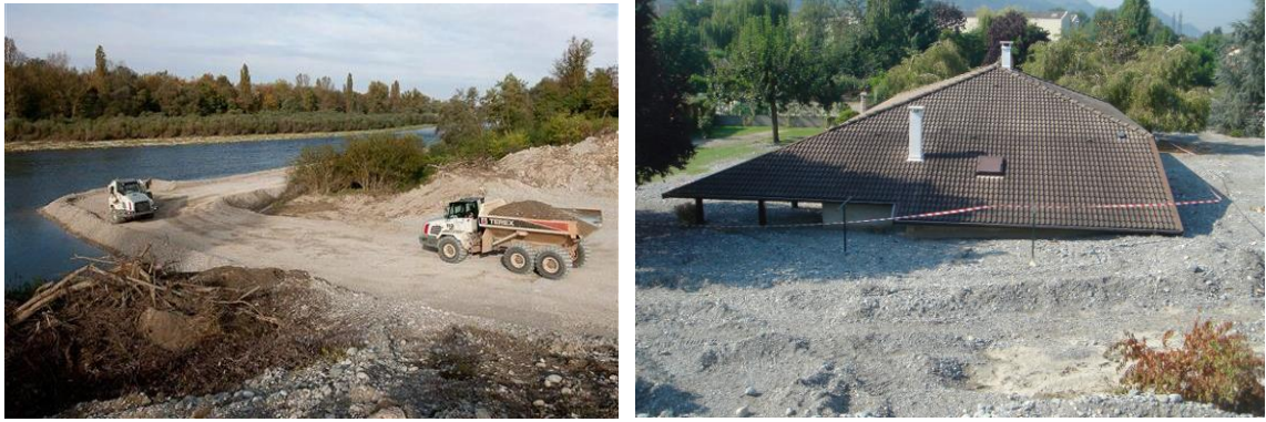
Figure 1: (a) Injection of 25000m 3 of sediments for ecological restoration of the Rhine River near Kemb (photo Alsace.fr) (b) Sediment deposition on the Domenon River and its impacts on population safety (Photo Belleudy)
