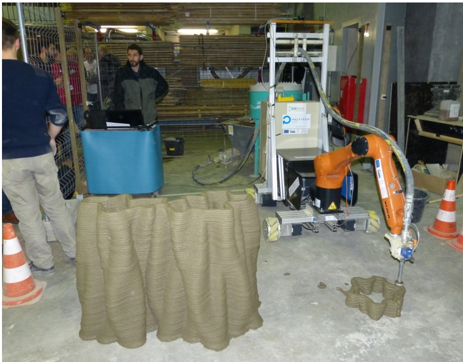
Figure A.18 – 3D printing during the results restitution evening on December 6, 2018 - Cement material form - ENSAPL
