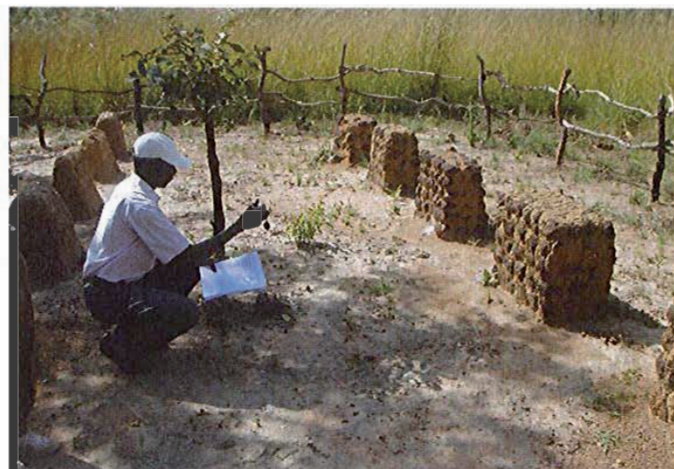
Fig.6 Preventive measure with sacrificial capping, Fayaz Tepa, UNESCO-Japan-Fund-in-Trust project, Uzbekistan (credits: Thierry Joffroy, 2003)
