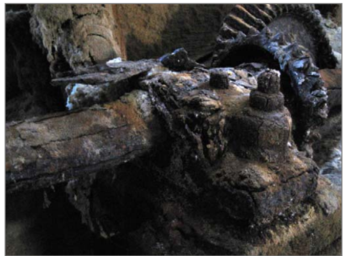
Figure 21: Photograph of bearing and distorted axes (2007)
