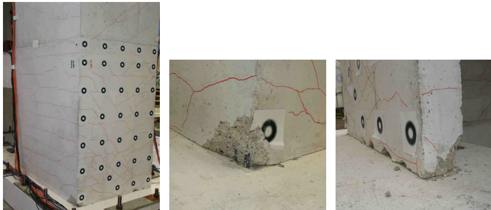
(a) Walls #1 and #2 — shear cracking. (b) Walls #1 and #2 — concrete crushing. (c) Wall #1 — transversal crack.
