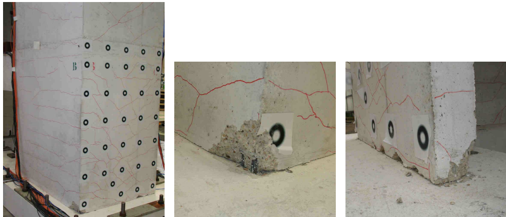
(a) Walls #1 and #2 — shear cracking. (b) Walls #1 and #2 — concrete crushing. (c) Wall #1 — transversal crack.
