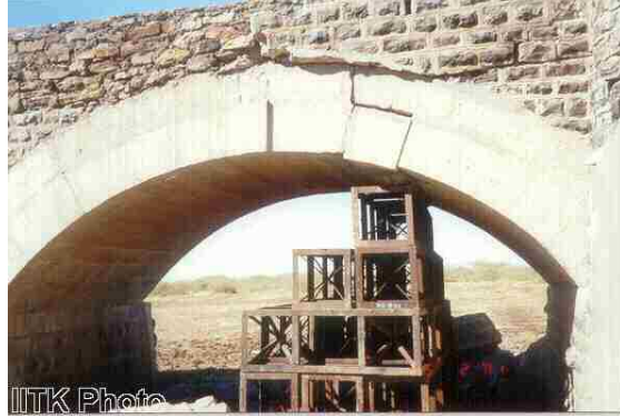
Figure 4.8: The stability of the bridge is compromised by the dislocation of one stone.
