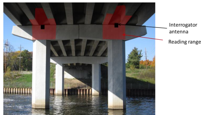
Figure III.7.1 Survey of a section of a concrete structure by using only one interrogator antenna (picture adapted from (Jansen, 2011)).
