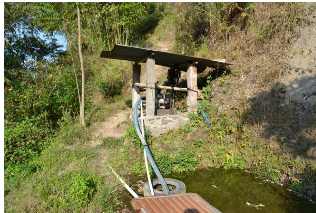
Figure D.3: Pumping system to bring water from the upper spring to the villages.
