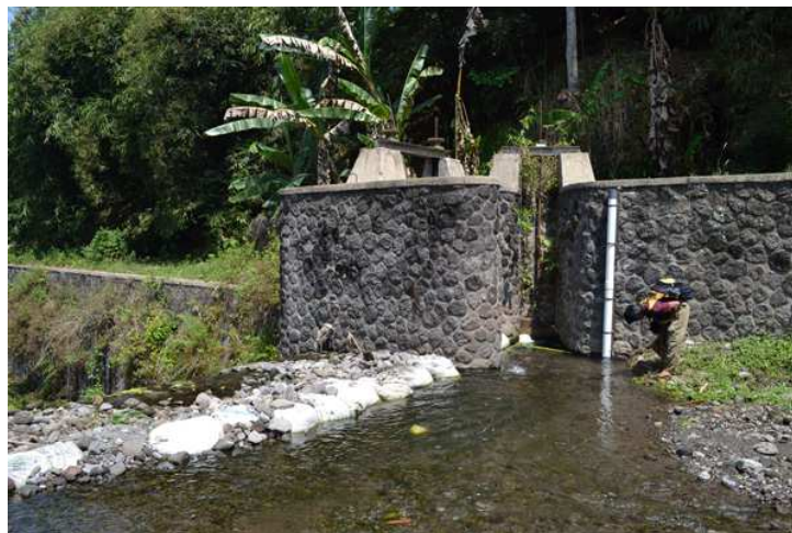
Figure 3.5: Automatic Water level recorder (AWLR) on the Pusur river at Kemiri dam (400 m asl). The floating system is protected from the solid discharge by a PVC tube (in white) and fixed on the dam's wall.
