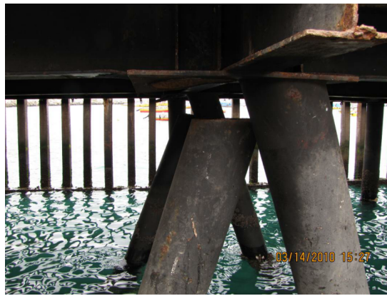
Figure 2.15: Port of San Antonio: Failure of the head connection between the wharf and the inclined piles after the Chile earthquake (after GEER [7])
