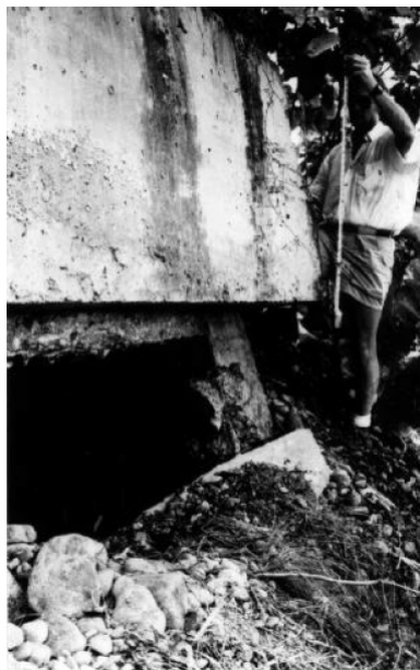
Figure 2.6: Rio Banano Bridge: Liquefaction induced rotation at the pile cap after the 1991 Costa Rica Earthquake (after Priestley et al. [5])
