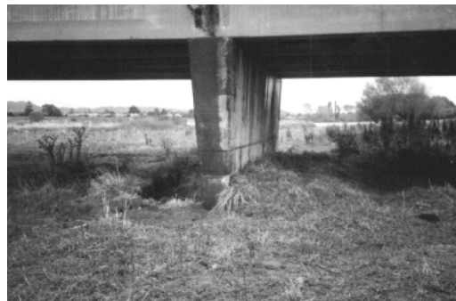
Figure 2.18: Pier C. The mound of the soil on the one side of the pier and the gap on the riverward side (after Berrill et al. [8])
