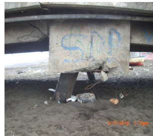
Figure 2.13: Port of Coronel: Damaged battered piles after the 2010 Chile earthquake (after GEER [7])
