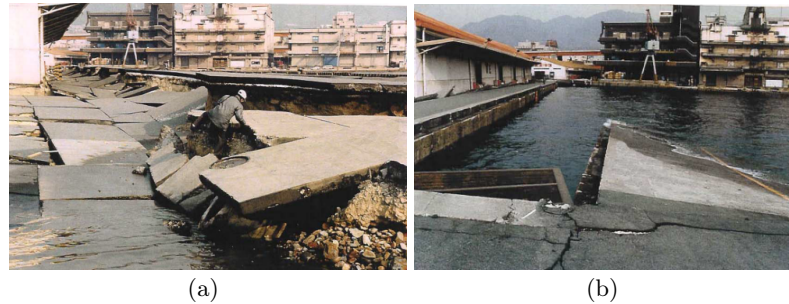
Figure 2.23: Post-earthquake observations of the severely damaged quay walls in Kobe earthquake
