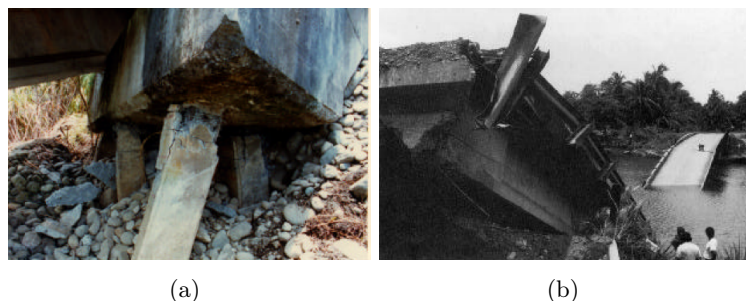
Figure 2.10: Rio Vizcaya bridge: (a) Damaged batter piles (north abutment); (b) Liquefaction failure mode of the bridge after the 1991 Costa Rica Earthquake (after Priestly et al. [5])
