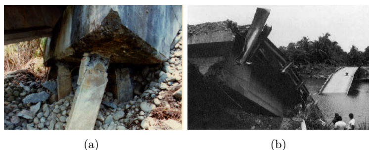
Figure 2.10: Rio Vizcaya bridge: (a) Damaged batter piles (north abutment); (b) Liquefaction failure mode of the bridge after the 1991 Costa Rica Earthquake (after Priestly et al. [5])
