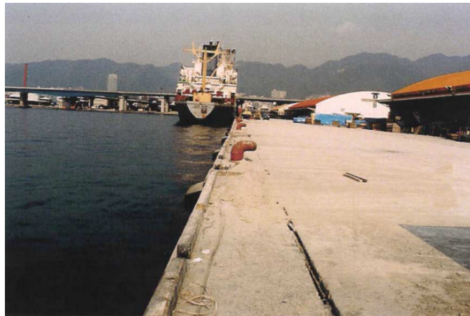
Figure 2.21: Post-earthquake observation of the survived quay wall in Kobe earthquake
