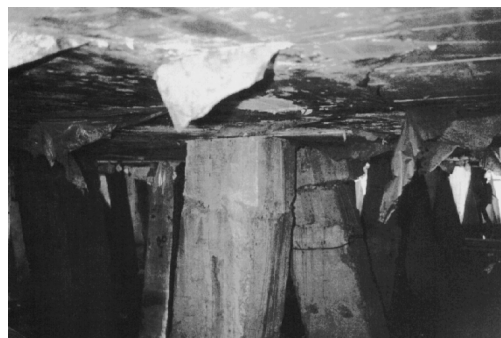
Figure 2.12: Container Terminal in San Pedrito: Earthquake induced damage on the batter piles of the wharf after the 1995 Manzanillo earthquake (after Ovando-Shelley and Pomo [6])
