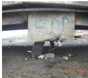
Figure 2.13: Port of Coronel: Damaged battered piles after the 2010 Chile earthquake (after GEER [7])
