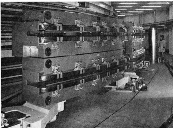
FIG. 4. — A bending-magnet installed in the DORIS-tunnel.
