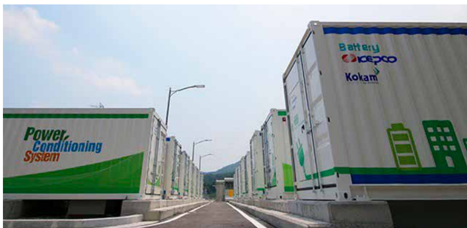
Figure 24 : Systèmes de stockage de l'énergie KEPCO (source : www.eqmagpro.com/kokam-to-build-36-megawatt-energy-storage-system-ess-for-kepcO-increasing-its-total-worldwide-ess-project-portfolio-to-132-megawatts-2/ )
