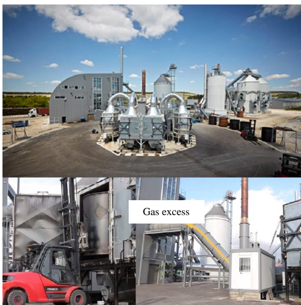
Figure 14. Carbonex technology overall view – unloading charcoal – cogeneration (France).
