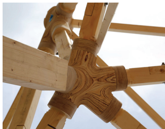
Figure 2. Photography of one out of 55 timber connection of the spatial structure, designed by URM MAP and manufactured by Stratoconception® additive manufacturing process. Photography by authors in Paris, La Vilette park, May 2024.
