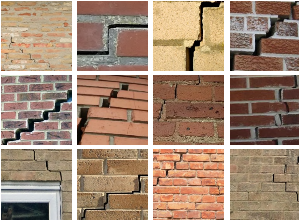
Figure 3: Examples of cracks in bonded masonry structures [5].
