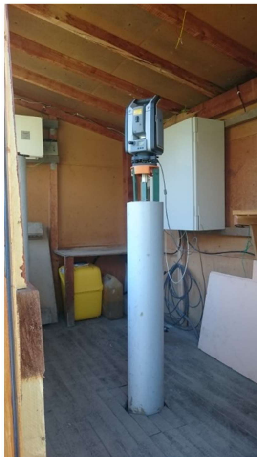
Figure 4. Permanent automated total station Trimble S9 Long Range on the pillar at the monitoring site at La Valette landslide (France)
