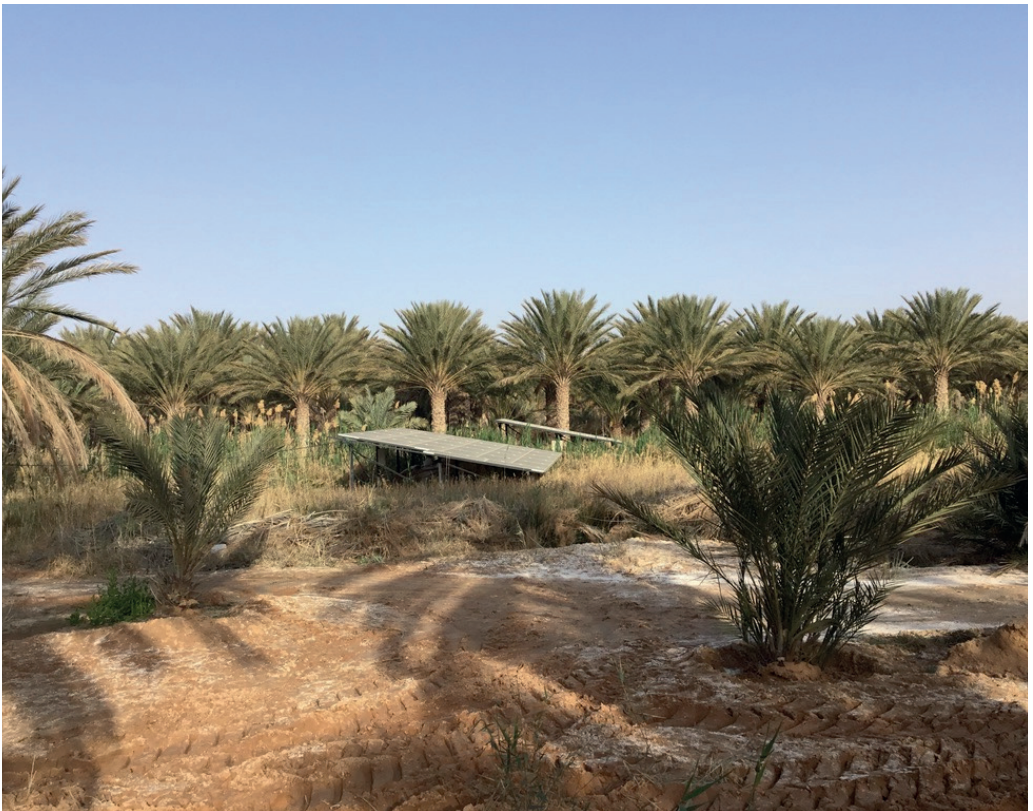
Photo 9. Solar energy system in palm groves in Kebili region
