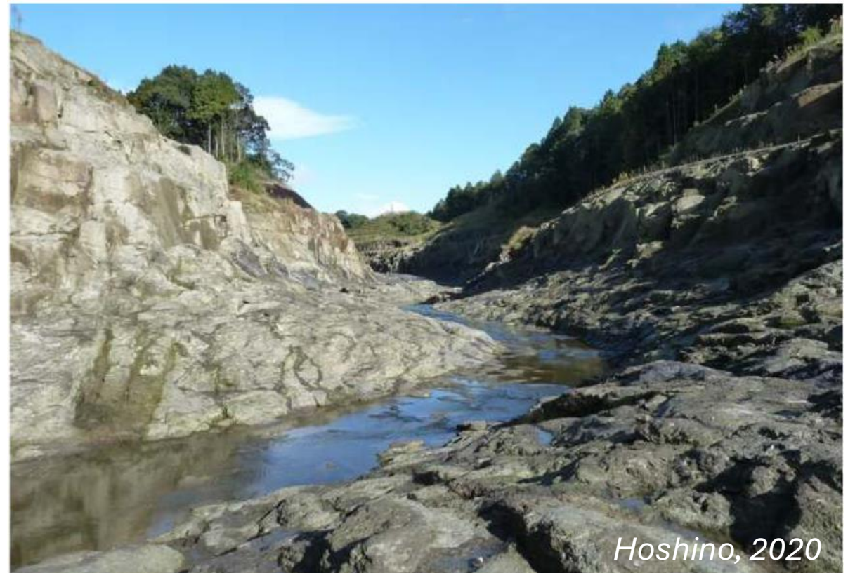
Canal of the Sogi waterfall just after completion of the work, Kyūshū
